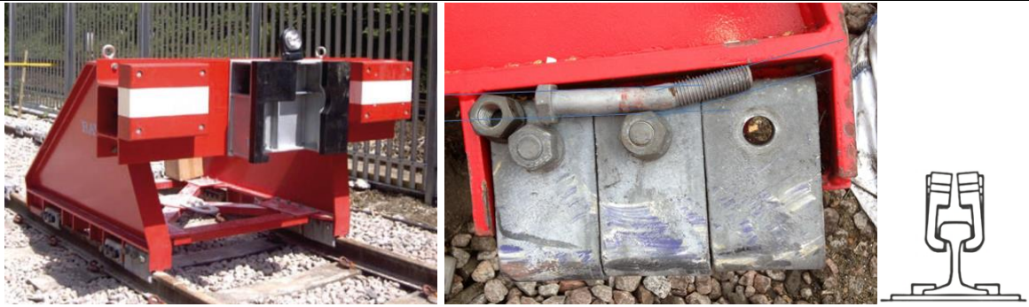
Figure 9 – Line buffer stop fails to arrest low speed train. Bent bolt indicates that bolt was not sufficiently tightened to provide clamping force. Bonus: crash assessment of train/buffer collision and structural repair of damaged bodyshell.
